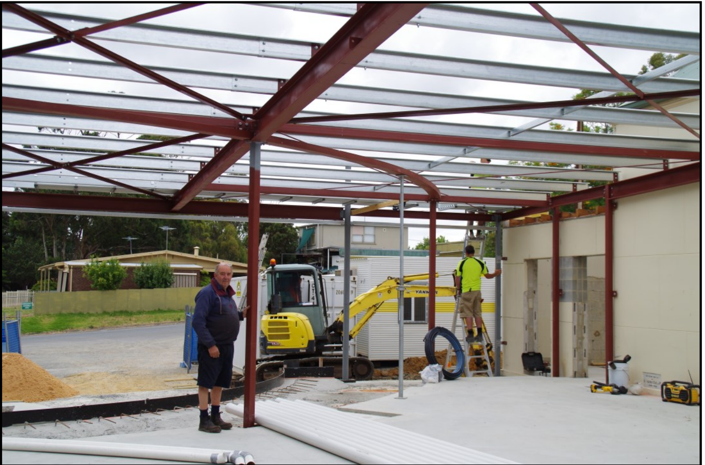
Above: Don Perry beside the new Hall Foyer framework that he constructed in 2015
